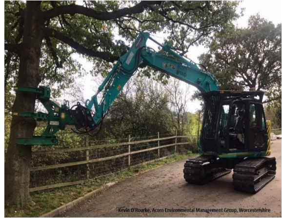
Fig 14: A tree shear mounted on an excavator or tractor can delicately extract trees from dense broadleaved woodlands
